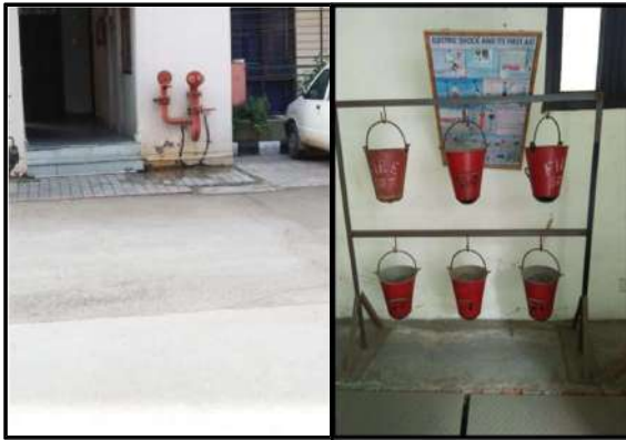
Fire Fighting Equipment
